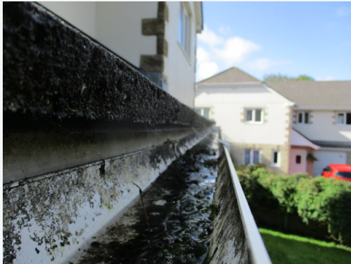
Front elevation ground floor gutter
