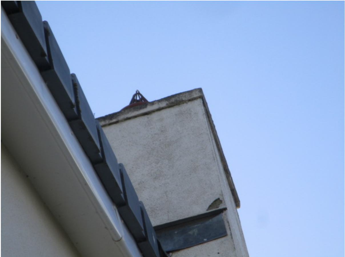
Localised render defect
